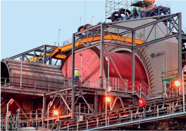
Stone mill in South Africa with large bearing operated via a central lubrication system. The oil volume is measured with VHS equipment of GHM.
