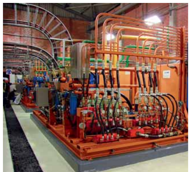
Central lubrication system with GHM Honsberg flow meter, Pressure sensors and temperature sensors.
