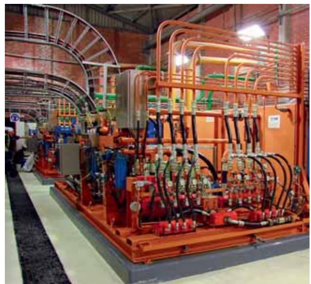
Central lubrication system with GHM Honsberg flow meter, Pressure sensors and temperature sensors.
